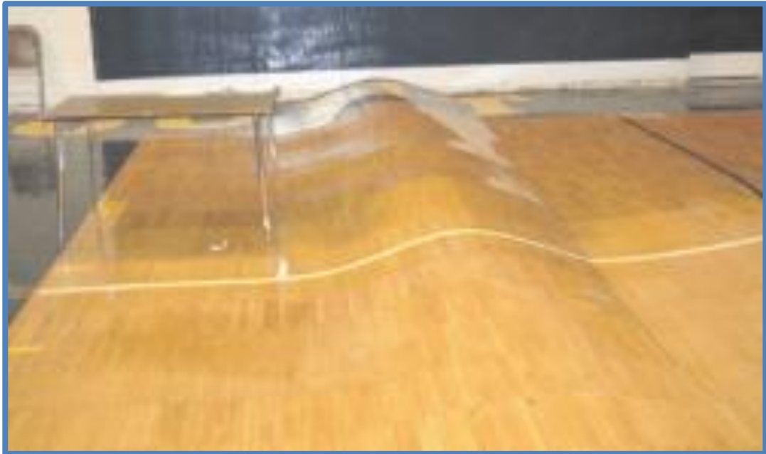
Cupping of the floor 3
